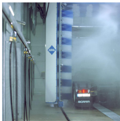
Hose-transportation in a truck washing facility
