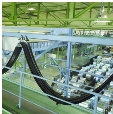
Energy and data transmission on a steel-mill-crane
